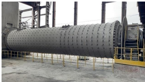
Figure 1. Cement tube mill 3,2x15 m
