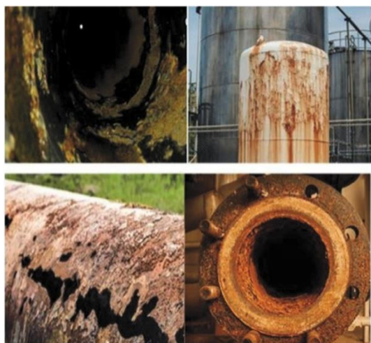
Figure 2. Different forms of Corrosion [45]
