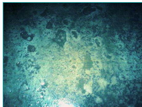
Figure 5 - Appearance of tank bottom section with visible thickness reduction due to corrosion
